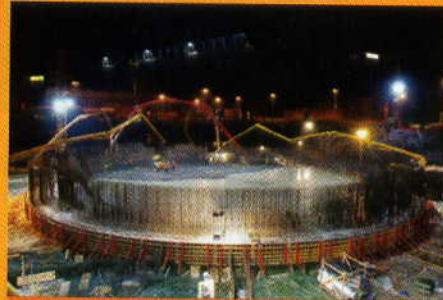
Under construction: an advanced (generation III+) 1,600-megawatt nuclear power plant in Olkiluoto, Finland.
